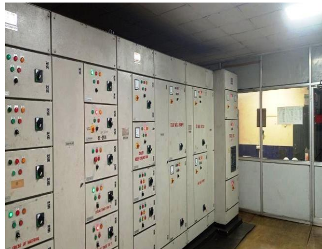
SLD Drive Room
