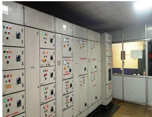
SLD Drive Room
