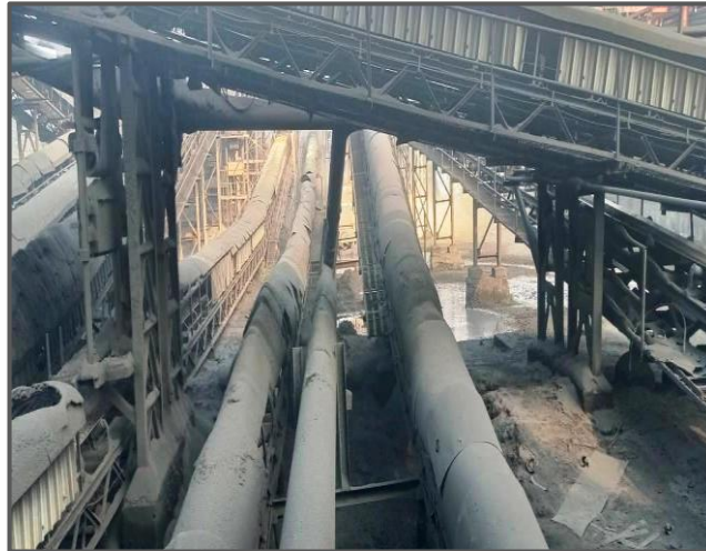
Conveyor For KILN
