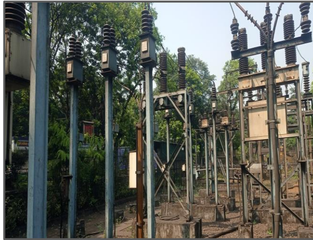
33 KV Bay Area
